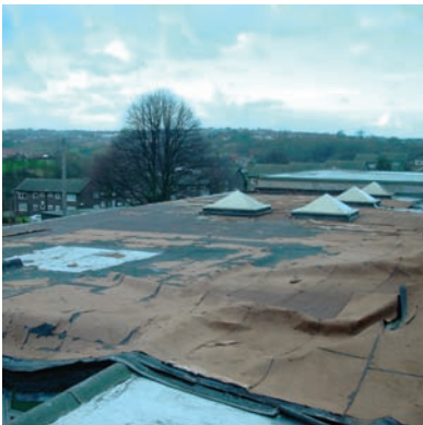
Wind damage resulting from poor design
