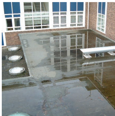
Ponding caused by poor design and maintenance
